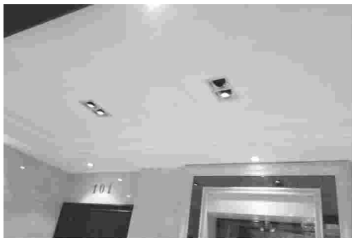
阴阳角方正，线条顺直
