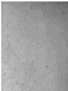
纵向贯穿性裂纹
